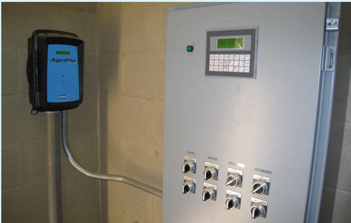
Figure 3: The Series3 MACE AgriFlo unit installed in the control "hut" and interfaced to a Modbus SCADA package that controls the piped off-take
